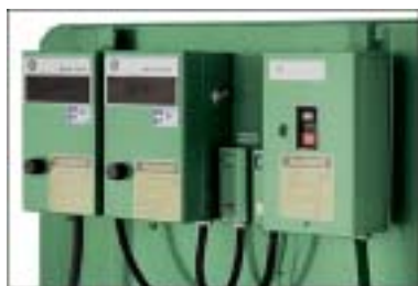
Starters shown mounted & wired.
